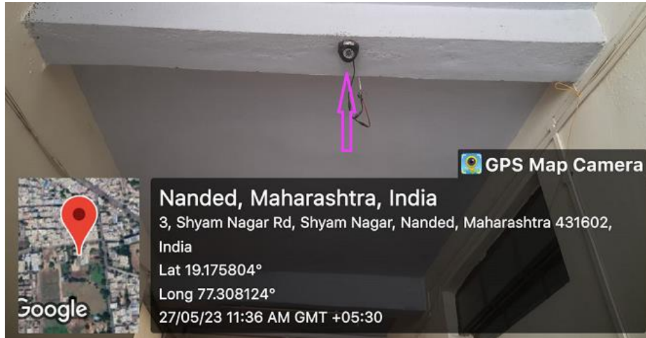
CCTV CAMERA IN CORRIDOR
